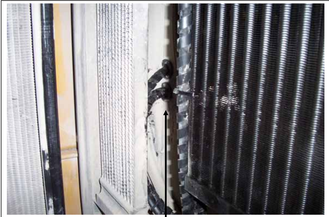
5/16" and 13/32" hose coming through the fan shroud.
